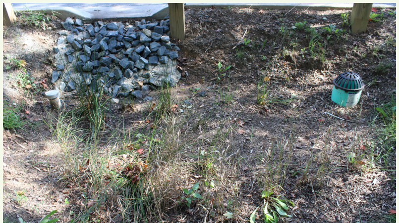
Micro-bioretention facility with sparse vegetation due to improper care during establishment
