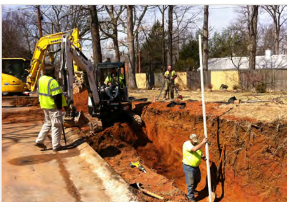
Workers excavate part of the Dennis Avenue right-of-way to make way for a bioswale.
