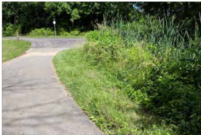
Figure 23. Current conditions of channel along trail. The area is overgrown with water tolerant plants.
